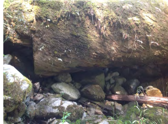
right bank of fill retaining log - not tied in very well
